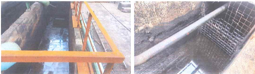
Drain leading to Buckingham Canal which was cleaned before inspection by CPCL
