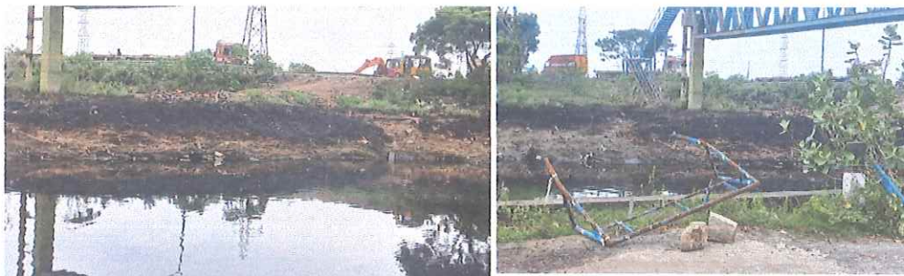
Oil Slick observed on side walls of Buckingham canal
