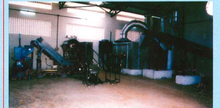
AUTOCLAVE & MECHANICAL LOADING INCINERATOR
