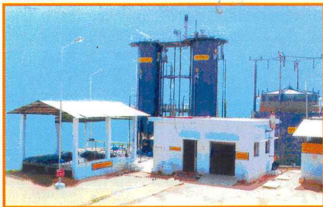
Bio Methanisation Plant in a CETP
