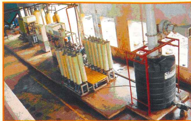
R.O.Plant - Disc Membrane
