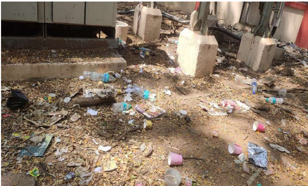
Figure 22. Generator area hotspot
