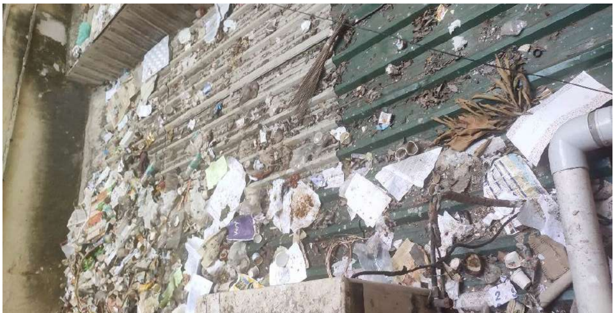
Figure 24. Littering on top of sheds
