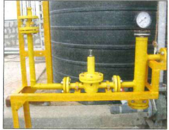
Fig. 4.6 Gas Chlorinator (Location 2)
