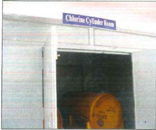
Fig. 4.17 Chlorine Cylinder Room
