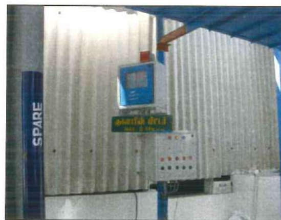
Fig. 4.24 Chlorine Alarm Device
