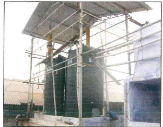
Fig. 4.10 Syntex Tank Chlorinator
