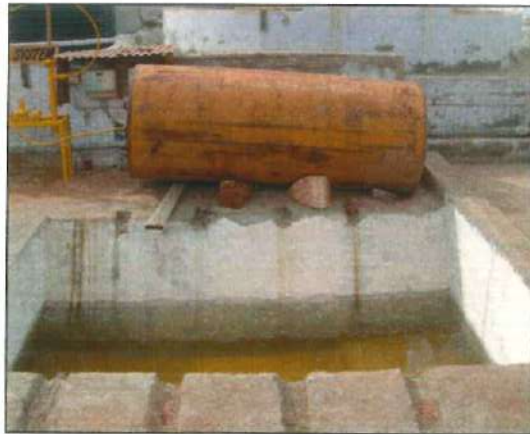
Fig. 4.27 Caustic Lye for Chlorine Absorption
