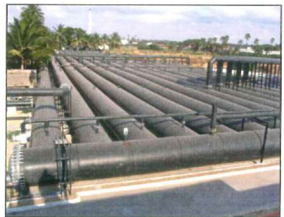
Fig. 4.16 HDPE Piping System as Chlorine Reactor
