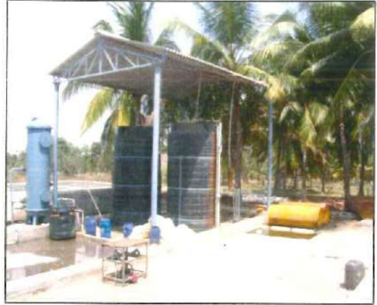
Fig. 4.18 Chlorine Tonners Exposed to Sunlight (Location 1)
