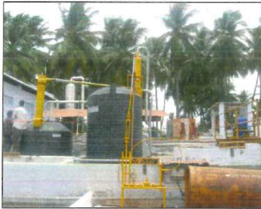
Fig. 4.13 Barometric Vacuum Break Loop (Location 3)
