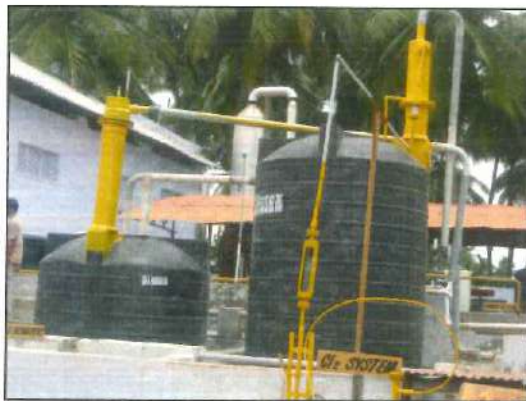
Fig. 3.3 Chlorination Treatment for Colour Removal
