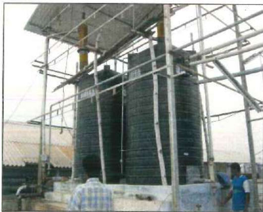
Fig. 4.11 Barometric Vacuum Break Loop (Location 1)
