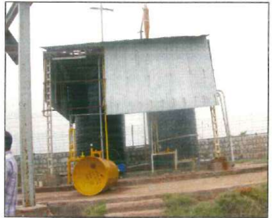
Fig. 4.14 Barometric Vacuum Break Loop (Location 4)
