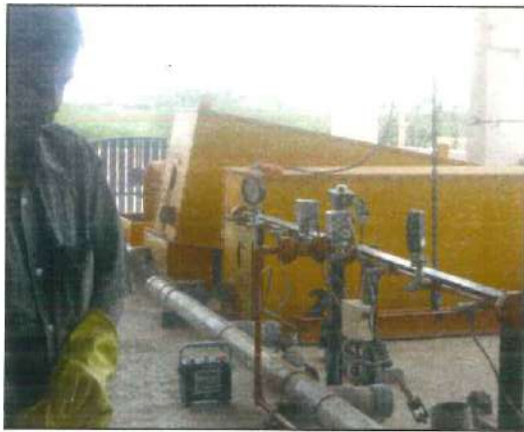
Fig.4.7 Gas Chlorinator (Location 3)
