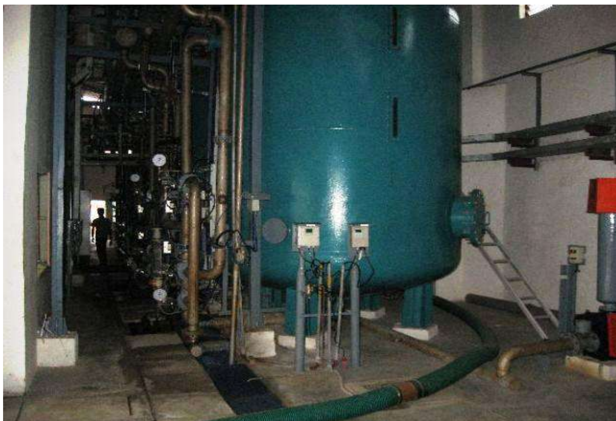
Fig. 7 Pre-treatment Unit (Filtration Section)
