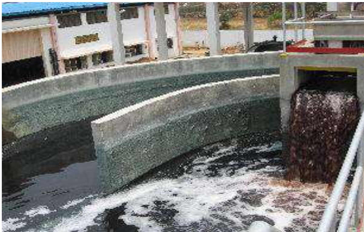
Fig. 4 Pre-treatment Unit (Storage and Homogenization Tank)
