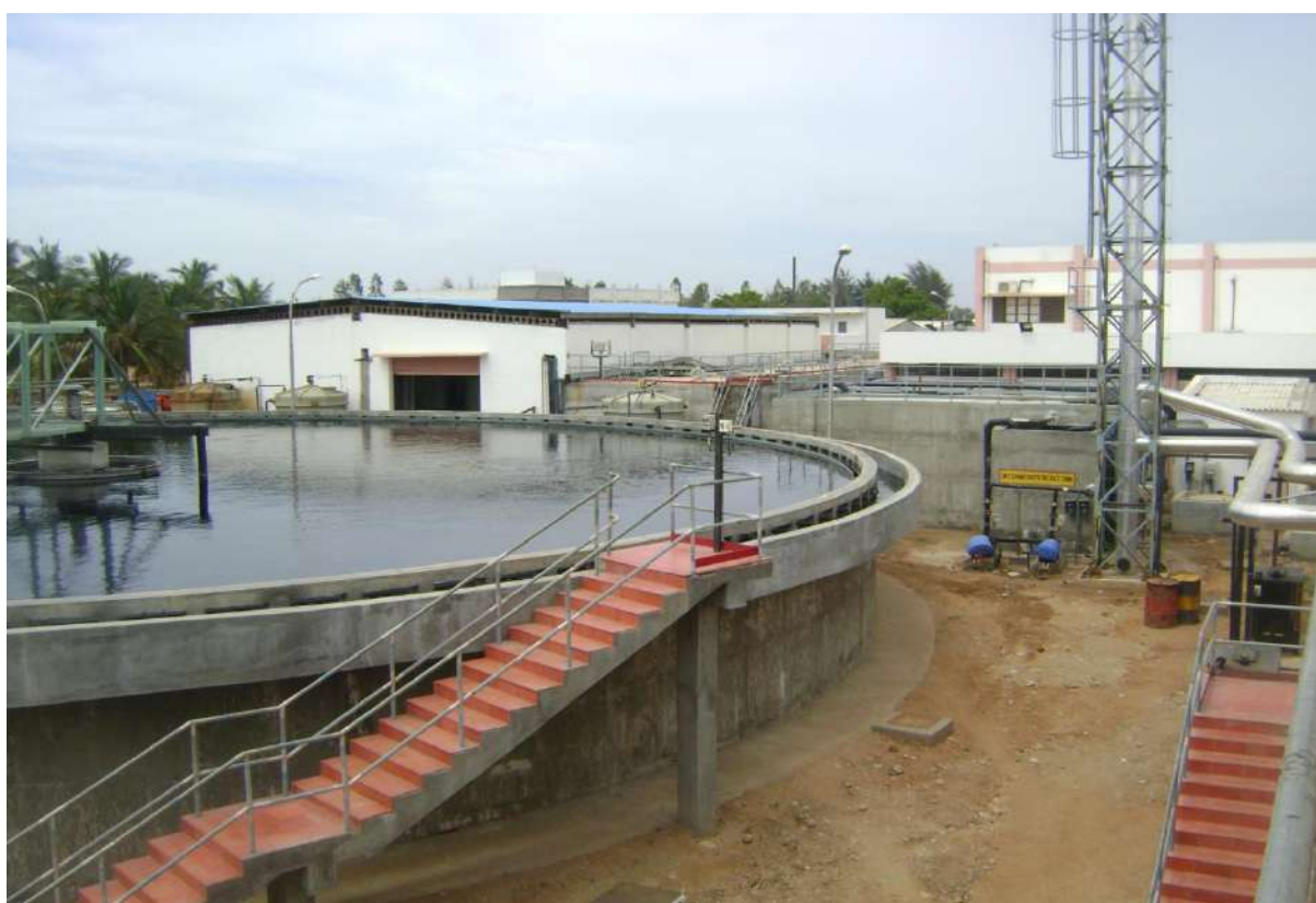
Fig. 6 Pre-treatment Unit (Secondary Clarifier Tank)
