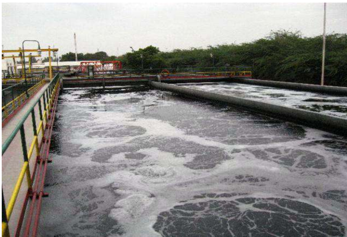
Fig.5 Pre-treatment Unit (Biological Oxidation Tank)
