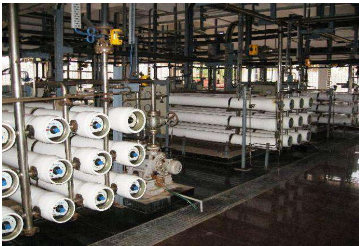
Fig. 8 Reverse Osmosis (RO) Plant
