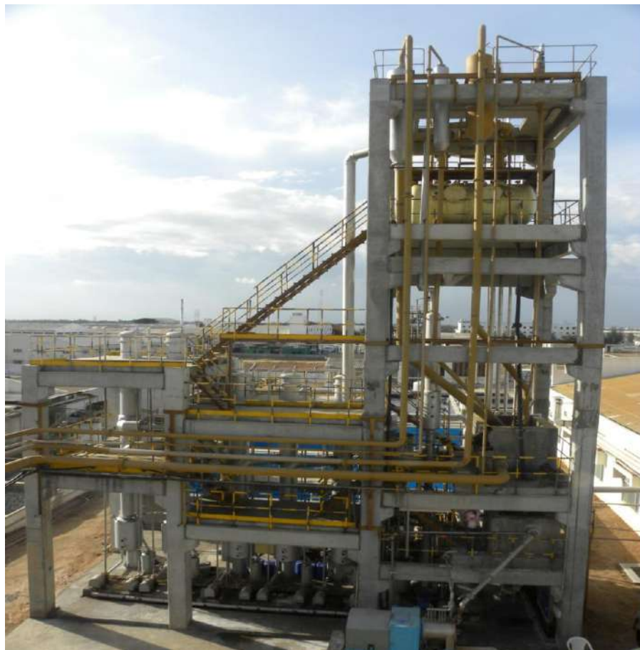
Fig. 11 View of Multiple Effect Evaporators
