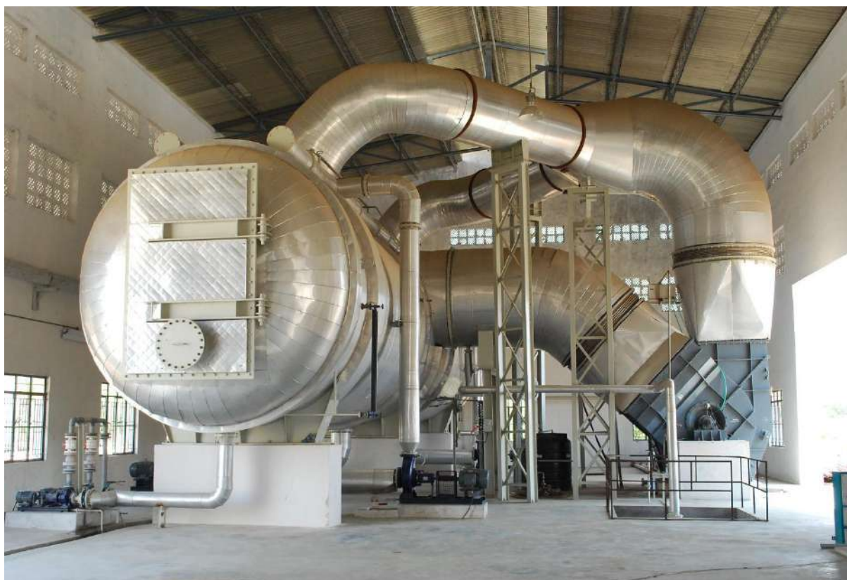
Fig. 9 Mechanical Vapour Recompression Evaporator Unit
