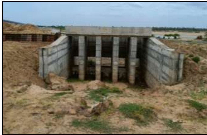
Fig No 1.1 Head sluice of north rajan channel
