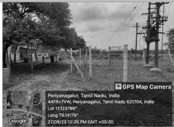
Figure 14. Electrical sub-station is installed in the West side of the proposed mine
