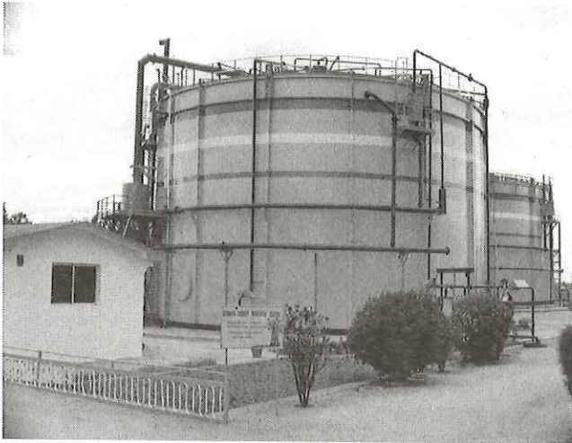
Anaerobic Bio-Reactor in Distillery
