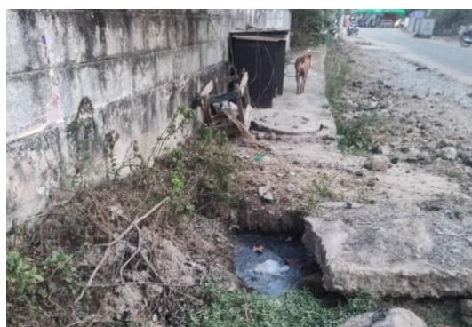
Figure 3-14: An open sewage in Manali, Chennai. (Source: FGD)
