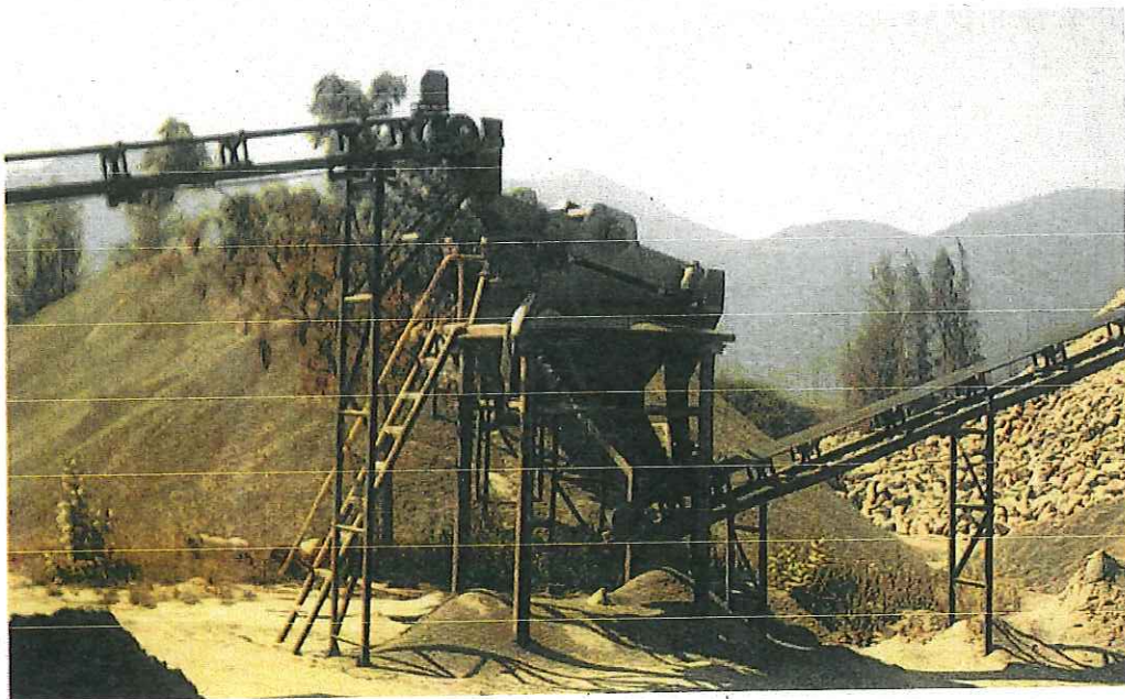
Additional Vibrator – (To segregate 1/2", Chips) – MS Cover
