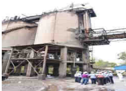
Figure 11 Silo for fly ash collection
