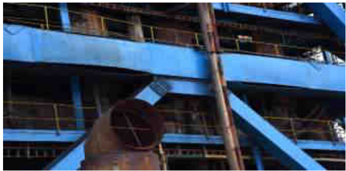
Figure 6 Damage to the girder
