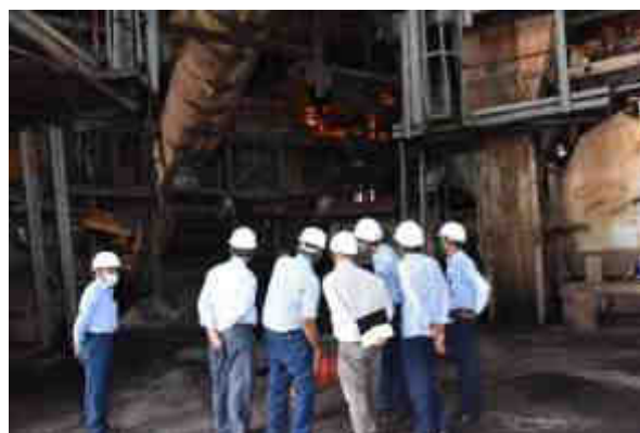
Figure 4 Slag conveyor and bottom ash collection point
