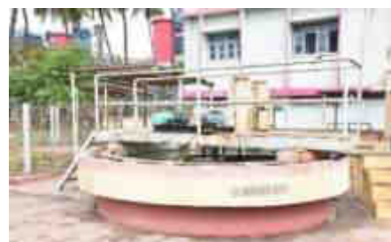
Figure 7 STP - Clarifier tank
