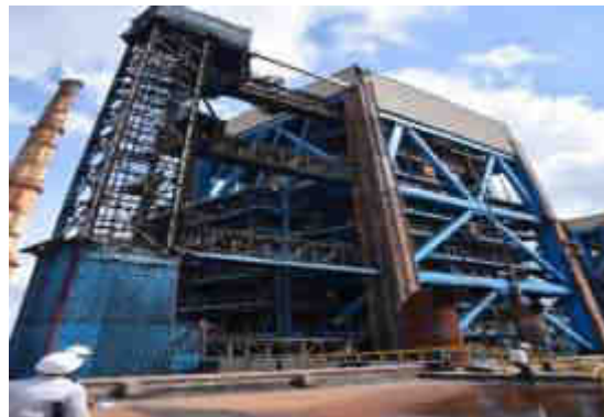
Figure 2 Steel structure supporting Boiler
