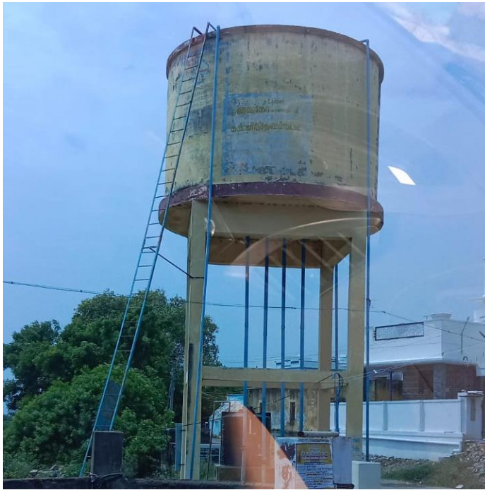
Water Tank - Gopalapuram
