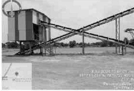
S5 – Crusher Unit (240m, N)
