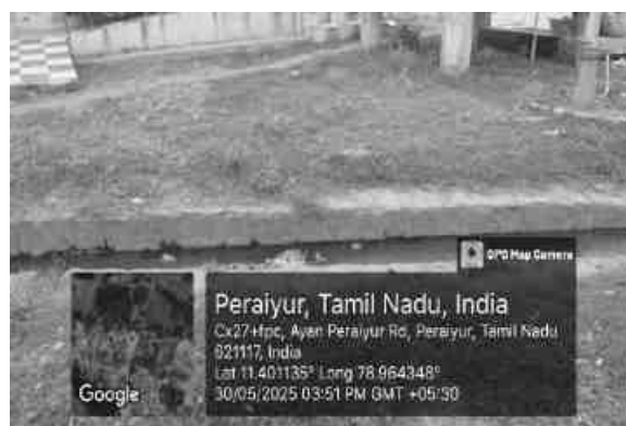
Open Drainage - Peraiyur
