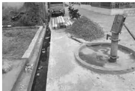
Hand Pump system – Devaiyur South
