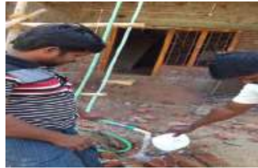
48, Perumal Sanathi Street, Bore well, Gopalamudram
