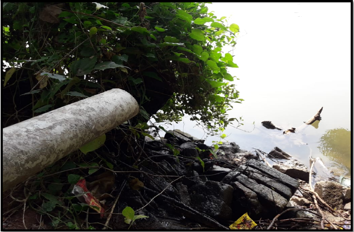
3. Pipe outfall near ARC Complex, Thiruvaiyaru.
