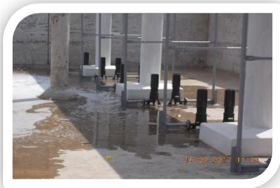
Original Hydro Dynamic Reactor- In Aeration Tank
