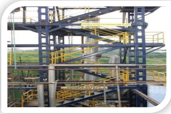
Double Effect Evaporation Plant
