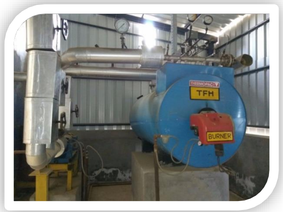
Thermic Fluid Heating System
