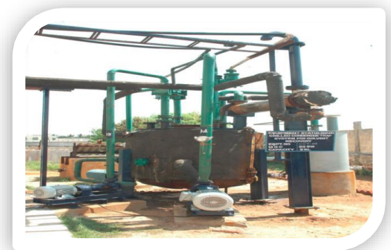
3 Stage HCL Scrubbing System
