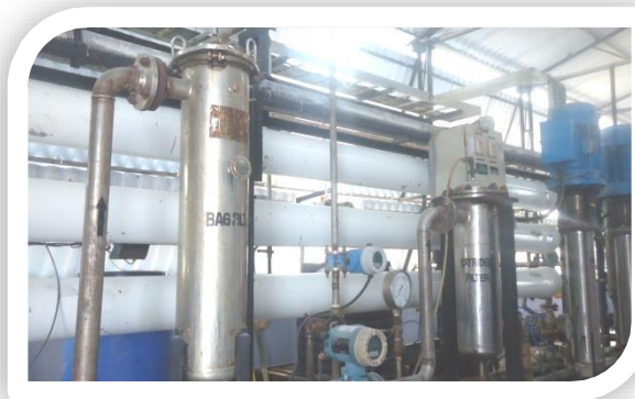
Flow Meters in RO plant
