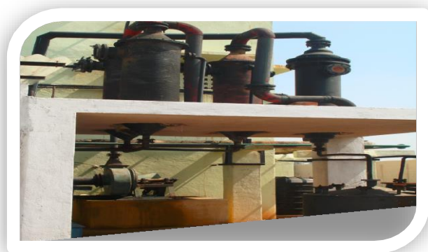
Chilled Condenser Trap System to Reduce Solvent Emission
