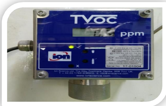
VOC Sensor at Paint Shop
