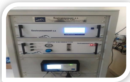
CSEMS - Thermic Fluid Heater Stack & Scrubber
