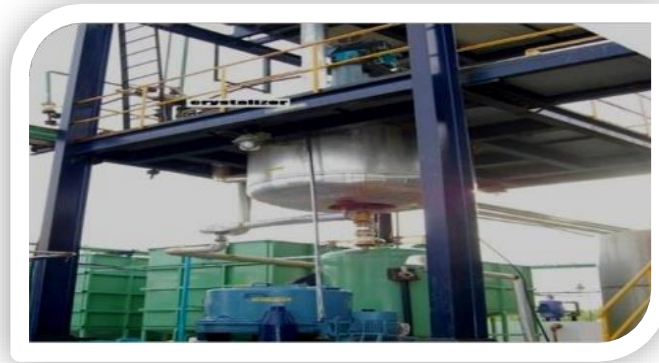
Forced Circulation Evaporation Plant
