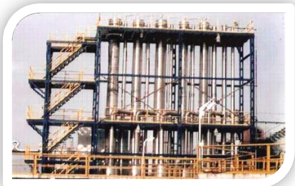
Multiple Effect Evaporator Systems
