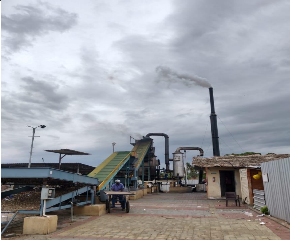
Incinerator for MSW functioning at Vairapalayam, Erode
