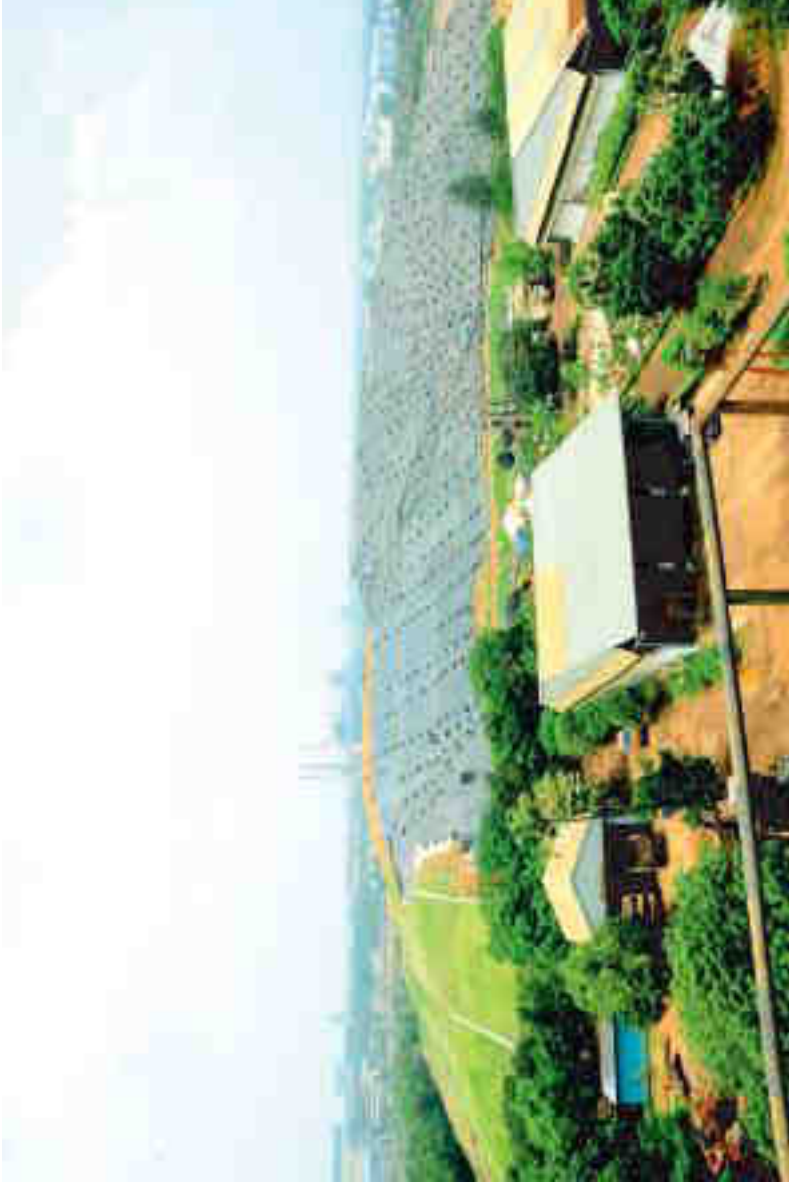
Aerial View of capping of hazardous waste secured landfill facility at Gummidipoondi.
