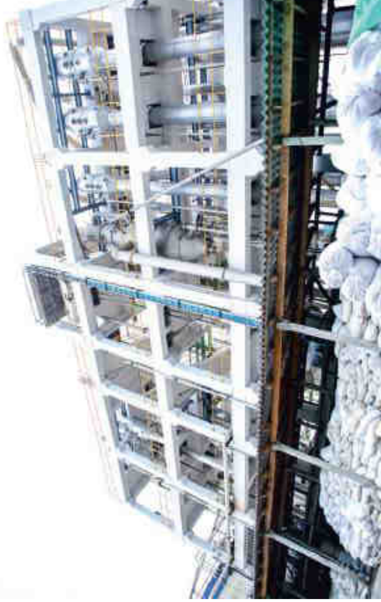
Multiple Effect Evaporator of a Textile CETP, Tiruppur with recovered salt
